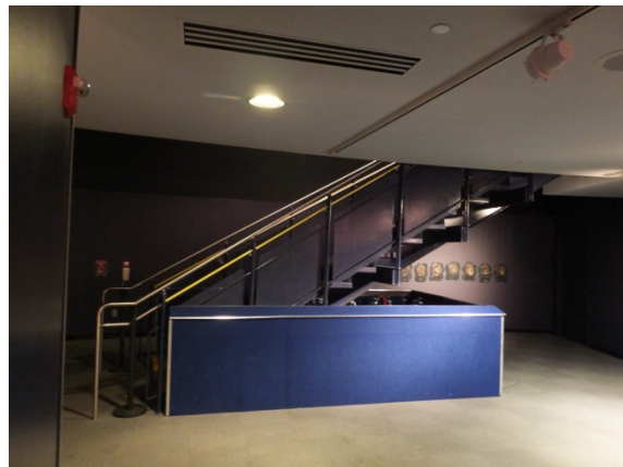
Figure 26. Underside of Stair Not Cane Detectable
