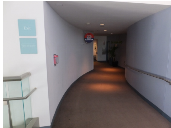
Figure 20. Ramp to OmniMax Lacks Handrail
